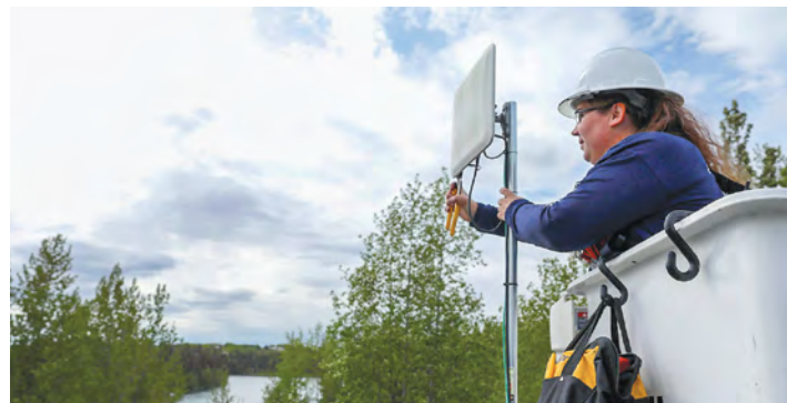
Top: Alaska Communications’ Daniel Rosin, left, and TJ Harvey install fiber-grade fixed wireless devices on the Kenai Peninsula. Above, Kristin Barber delivers broadband services in Sterling, an underserved community. All three are Anchorage Local 1547 members.
