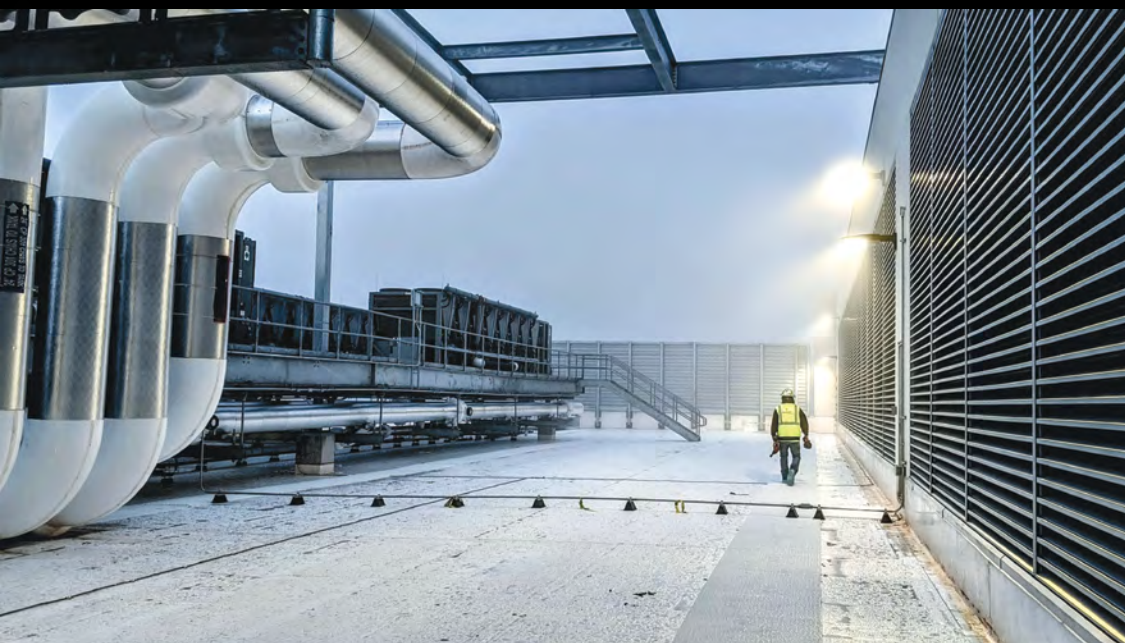
IBEW construction members are working on projects now, like this data center, worth $650 billion. In the next year, Projects worth another $800 billion are expected to start.
